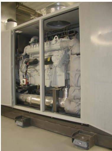
Detail on Combined Heat & Power Plant.
