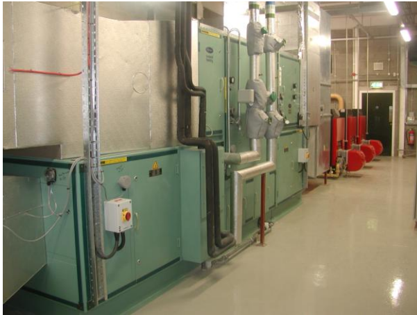
Detail of Air Handling Unit with Heat Recovery
